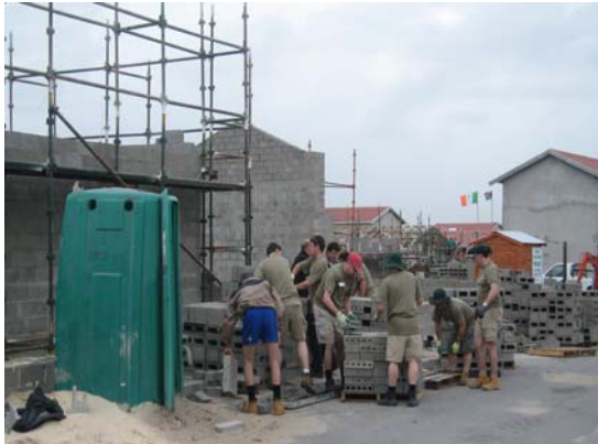
Diarmuid Gavin, TV celebrity gardener (pictured centre back) supervises construction of the Garden of Hope and Community Centre
